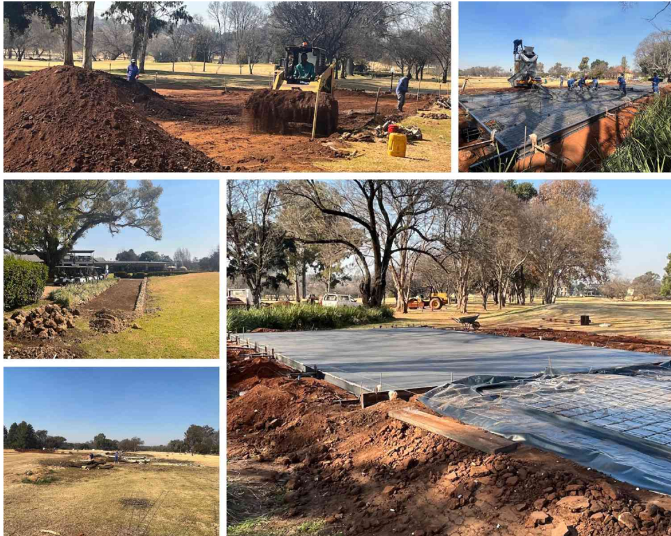
Clockwise from top left – padel courts being levelled, concrete being poured on the range, last tree cut down for the range and new pathway being prepped for the carts.
